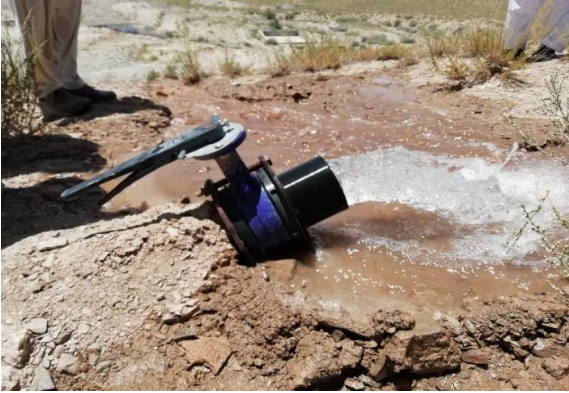
Provision of irrigation water through Pipe lining in command area of village Karr
