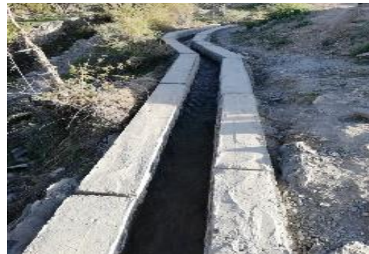
Construction of water course with stone masonry lining techniques was constructed successfully in VO Tor Tangai
